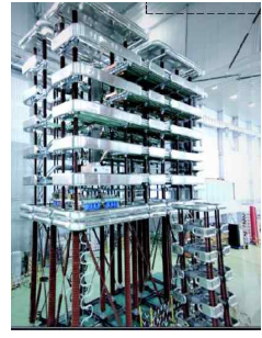
500kV DCCB (SGCC)
