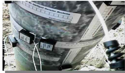
Multiple M2 Sensors fitted to subterranean Pipeline Prior to coating reinstatement and back filling
