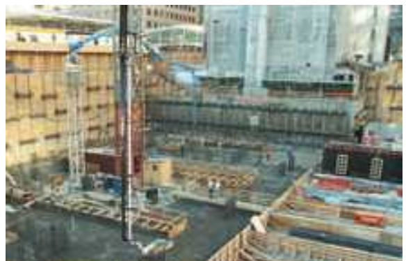
(b) Courthouse Concrete Footing, Canada, FA 50%
