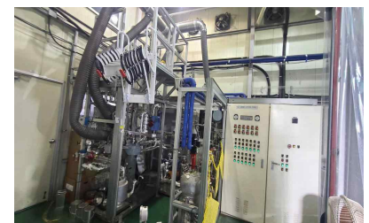
<SDA (Solvent Deasphalting) 설비>
