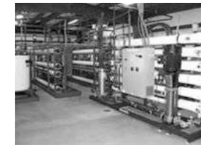
(a) Membrane ultra-filtration unit
