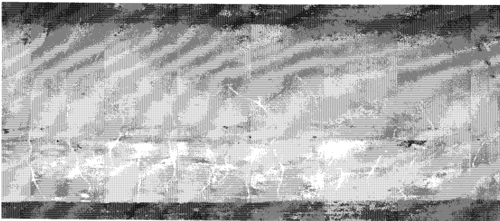
(a) exterior girder in span-1, seriously damaged by proof loading test
