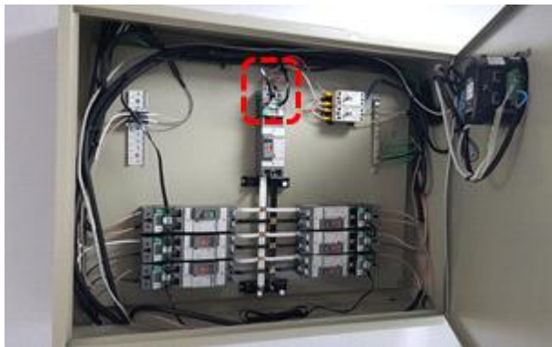
<Grid - Power Meter>
