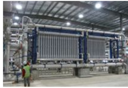
(b) Membrane ultra-filtration unit
