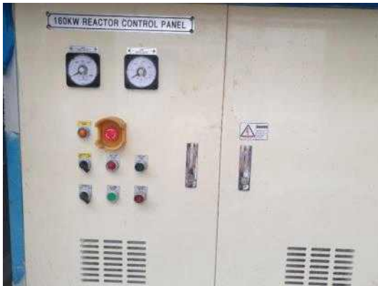
Reactor Control Panel
