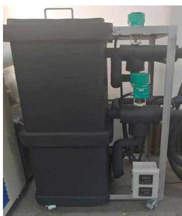
(b) Buffer tank 및 3-way 밸브
