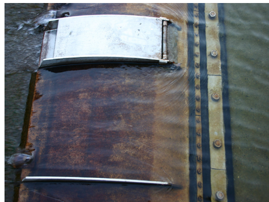
(b) Corrosion of steel materials
