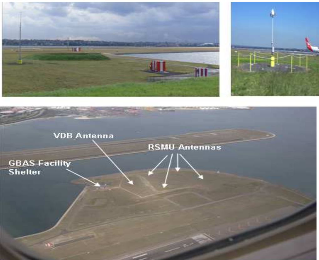
Sydney SLS-3000 GBAS Installation
