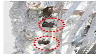
(f) Re-bar failure of K-RC-H
