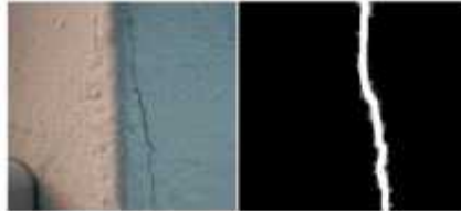
(Fig. 8) Masking of cracks using crack images
