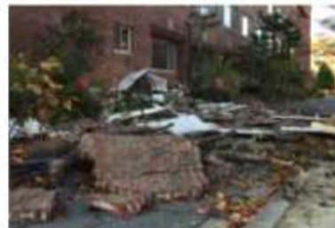
(Fig. 1) Failure of the masonry walls
